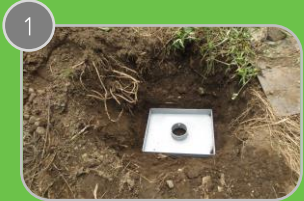
1 Dig hole and place the base plate at a depth of 300mm
